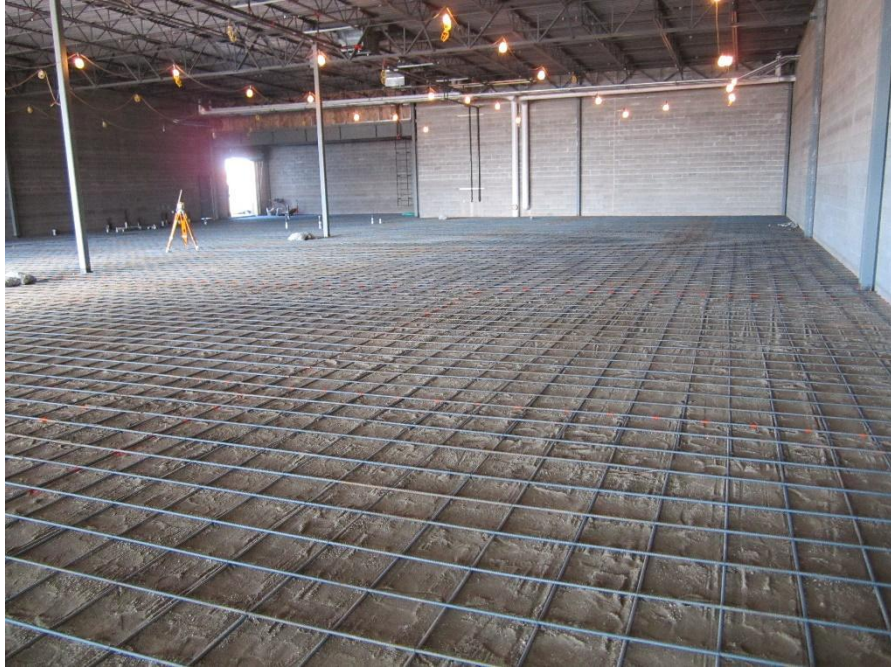
Figure 3. Rebar is laid down systematically to provide tension support for the concrete that will be poured over it. Once the concrete is poured, the rebar will take on most of the weight and ensure that the concrete will be a reliable, structural base. (This image was retrieved from Medford Concrete Contractors.
